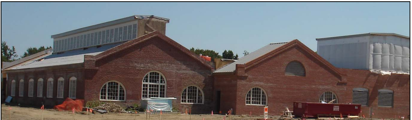
Coping and Marble Shop becoming part of South Section of Jay Hoffman Center at Nelson Campus of LCCC.
