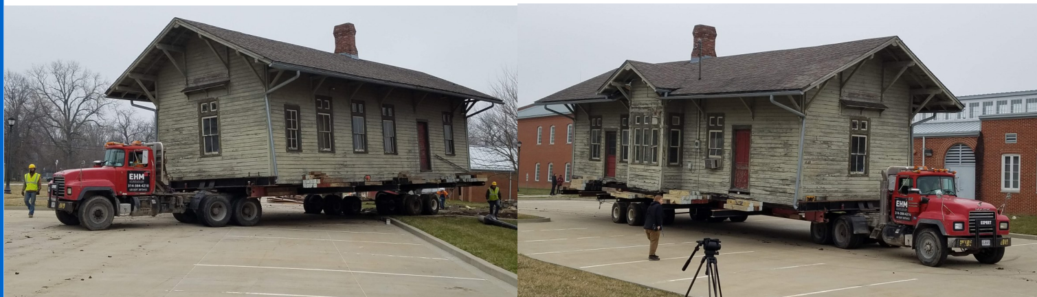
The 1883 Nickel Plate Station as it is moved to its new location. (Photos by Cindy Reinhardt)
